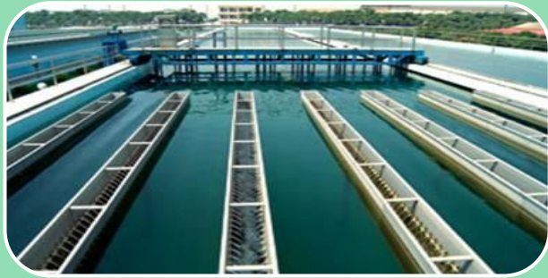
Water supply sanitation and quality maintenance
